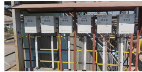
Renovation of sulfuric acid addition system at CNMC's Luanshya Muliashi hydrometallurgy plant
